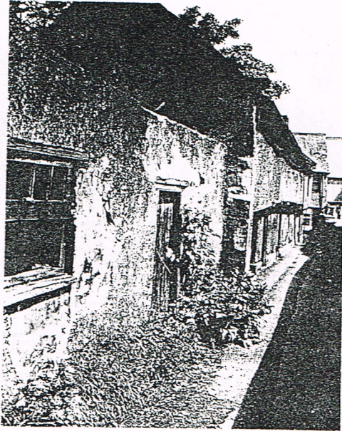
The South side of the structure, photographed in the early seventies. 28mm lens.
